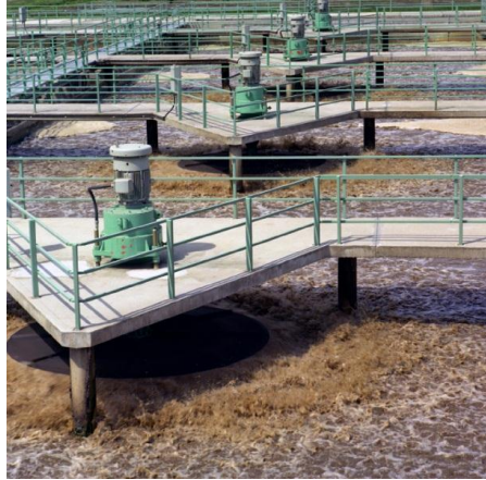
A sewage treatment plant
